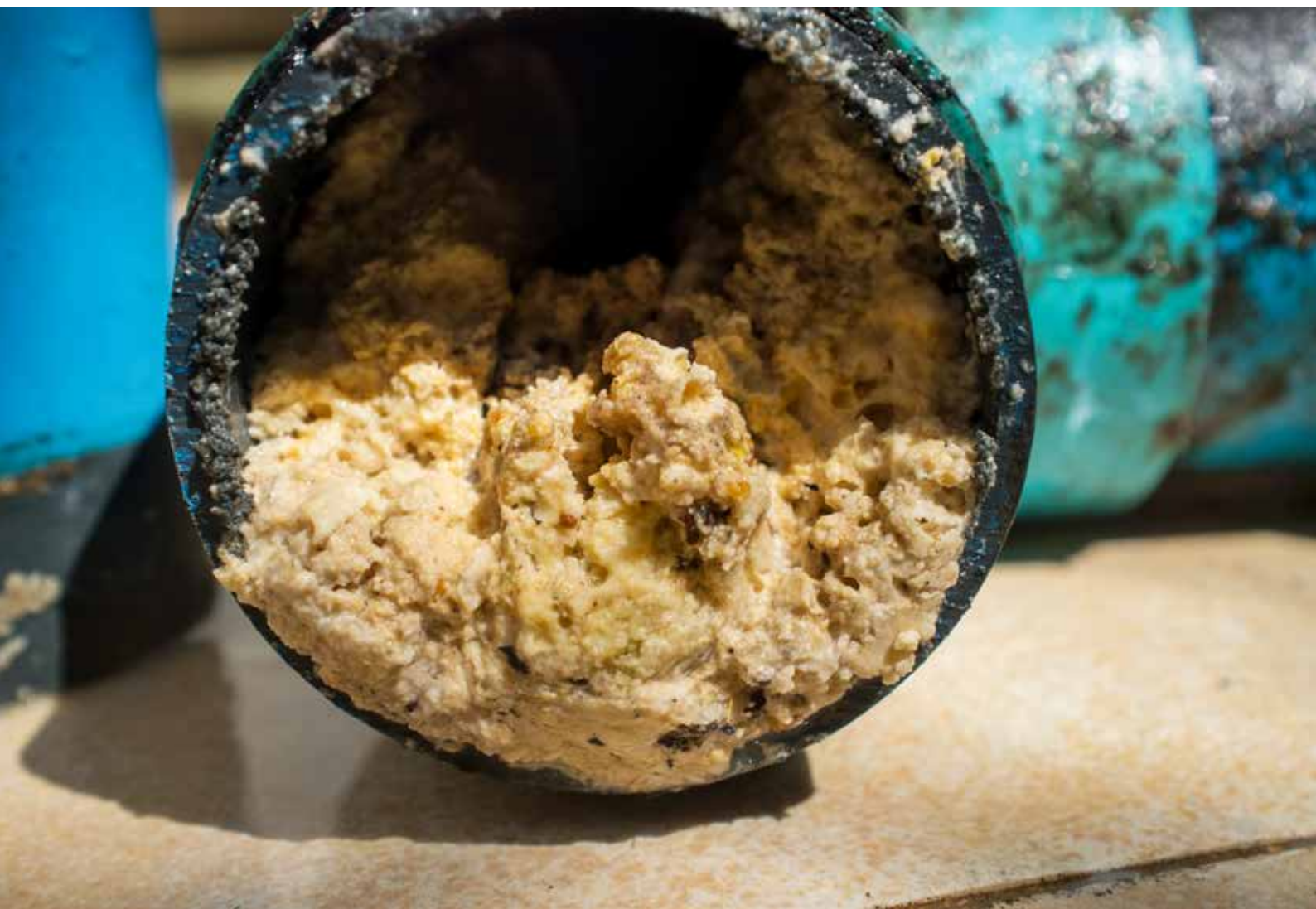
A pipe clogged with fats, oil and grease, nicknamed the “fatberg”, was found blocking a London sewer.
